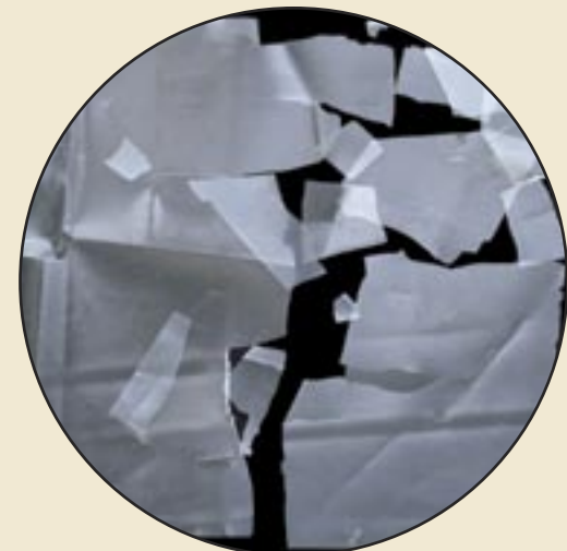
A sample of a deteriorated vapor barrier removed from a building.
